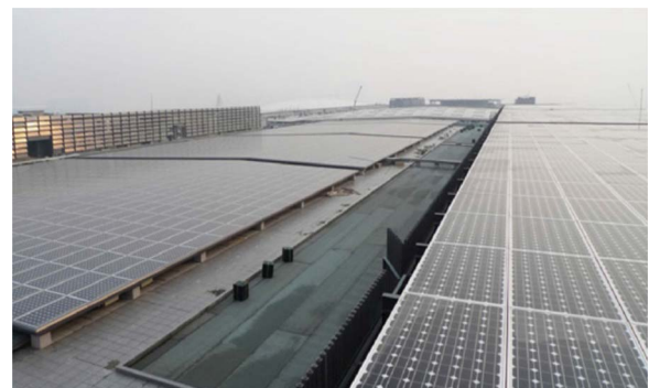
Fig. 2. Building Added PV system.
