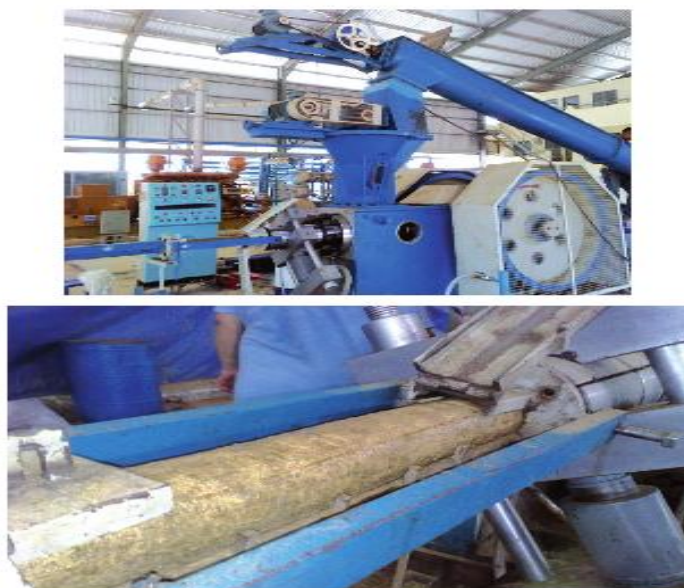
Figure 2.4: Piston press technologies in the production of palm biomass briquettes
