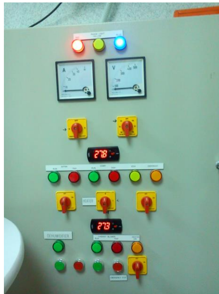
Fig. 2: Environmental chamber main switch controller
