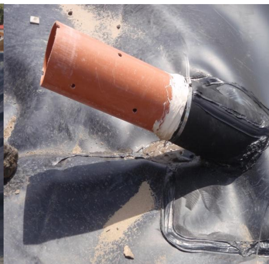
Figure 3.5: Methane collection drain pipe
