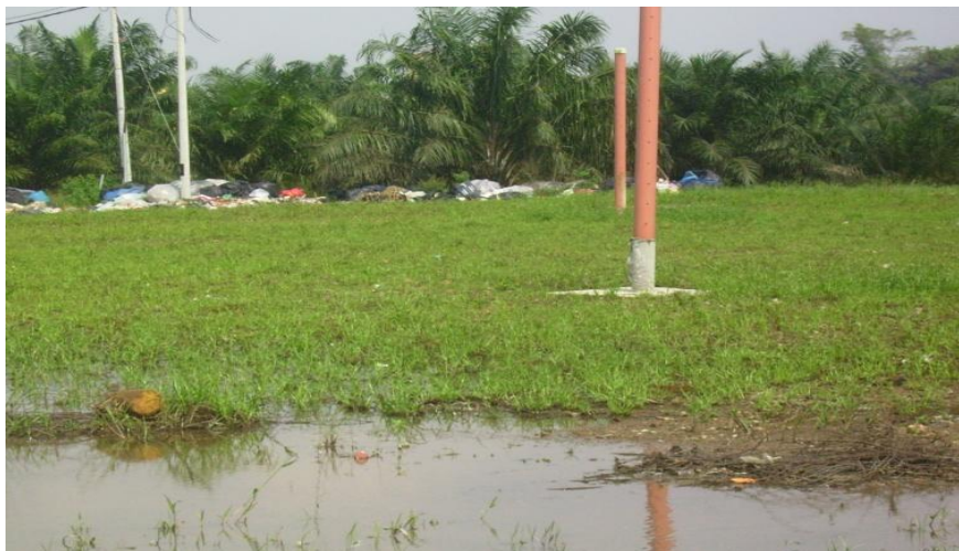
Figure 3.6: Methane gas drain from the old MSW landfill
