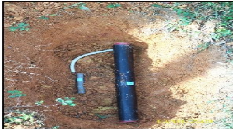
Figure 3.8 Cathodically Protected Coated Steel Pipe with Mg
