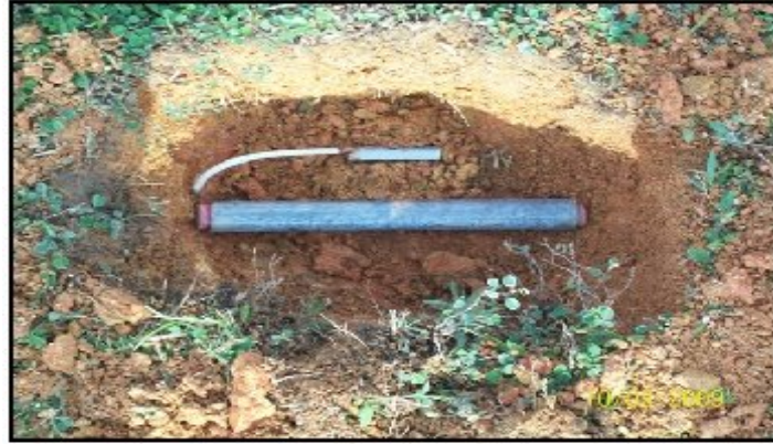
Figure 3.12 Cathodically Protected Uncoated Steel Pipe with Zn
