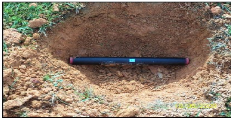
Figure 3.10 Unprotected Coated Steel Pipe
