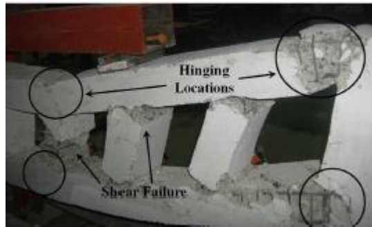
Figure 2.5: Failure mechanism of beam with square openings (Aykac et al, 2013)
