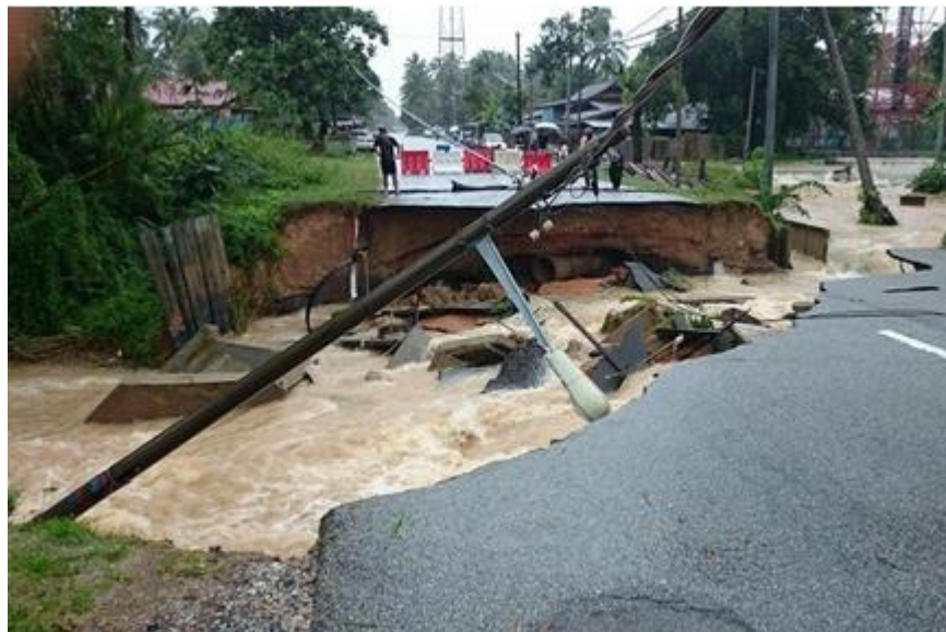
Figure 1.2 : Road damaged due to floods.(December 2014)
