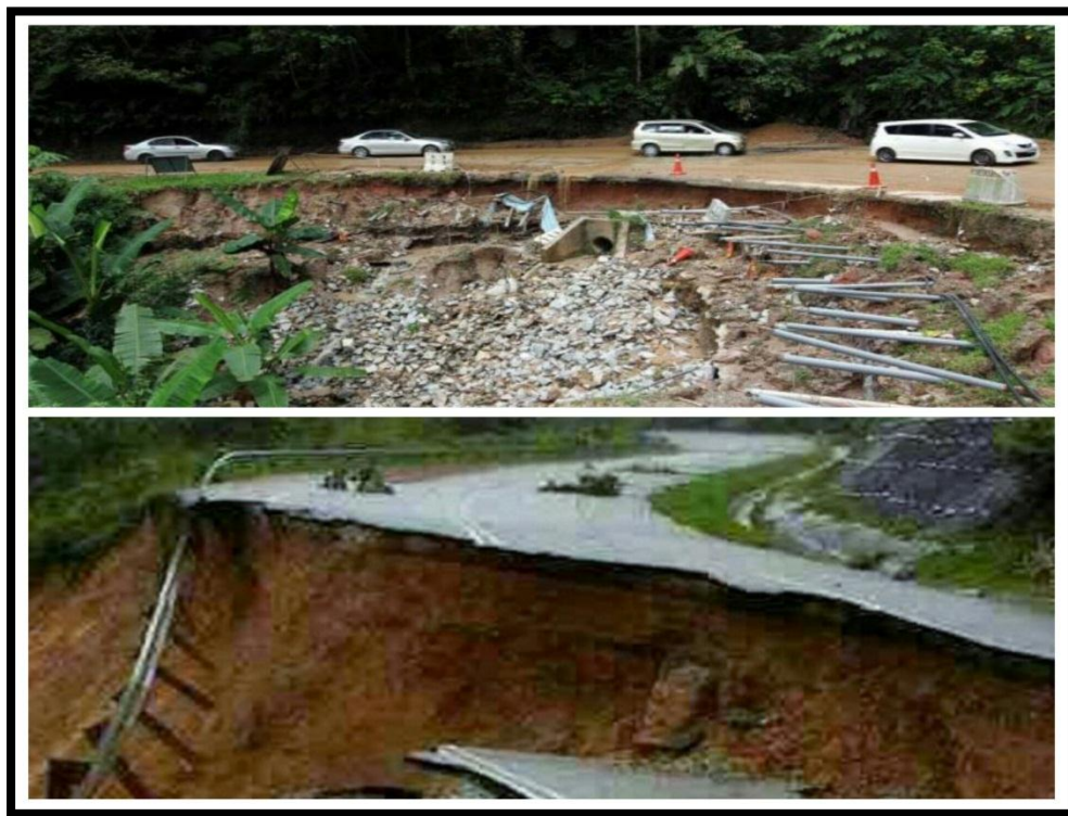
Figure 1.1: The damage Due to Landslide
