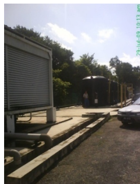
Figure A-15 : Machine that used in sewage treatment plant
