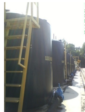
Figure A-16 : Sewage sludge tank
