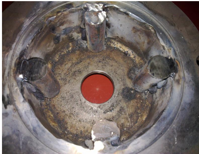
Figure 3.23: The mild steel rod have been welded on the turbine runner cover.
