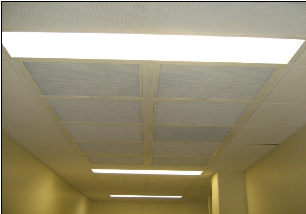
Figure 4. Lamps in corridor.
