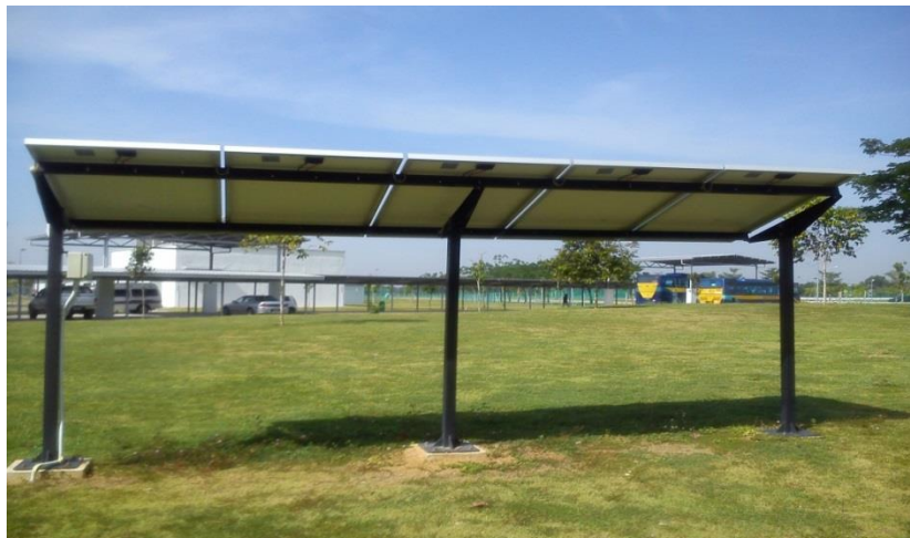
Figure 4.8 Solar Panel at Pekan Campus
