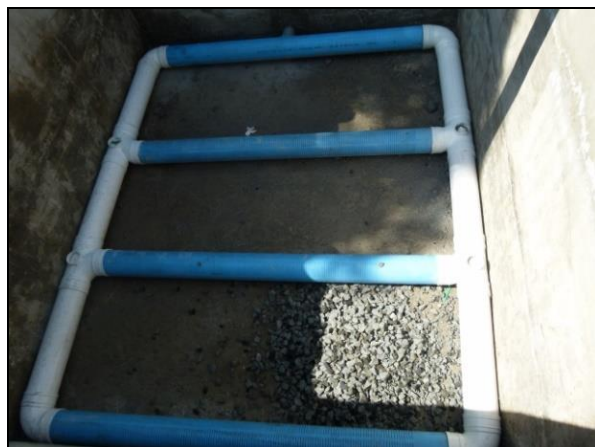
Figure 2: Self-made strainer using 4 inch uPVC screen pipe, uPVC pipe and uPVC connector
