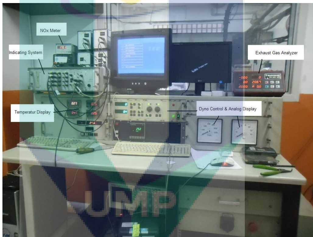
Figure 3.5. Instruments in the control room.
