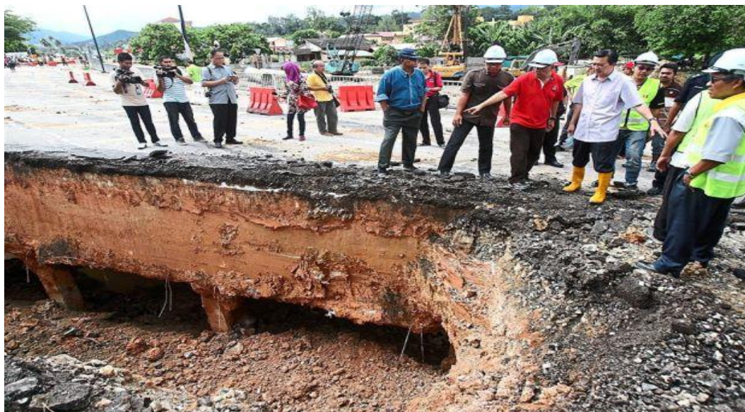
Figure 2.1 Damaged Kampung Baru Bentong bridge
