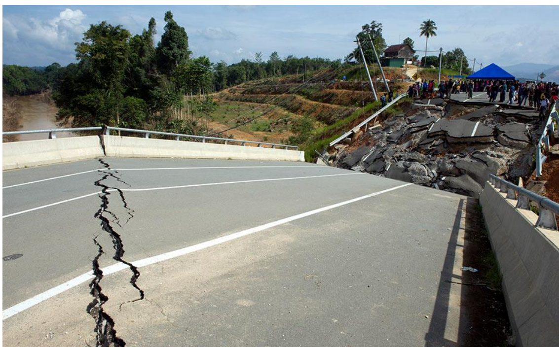
Figure 2.5 Condition Sungai Tanum bridge , Kuala Lipis , which was badly damaged by floods
