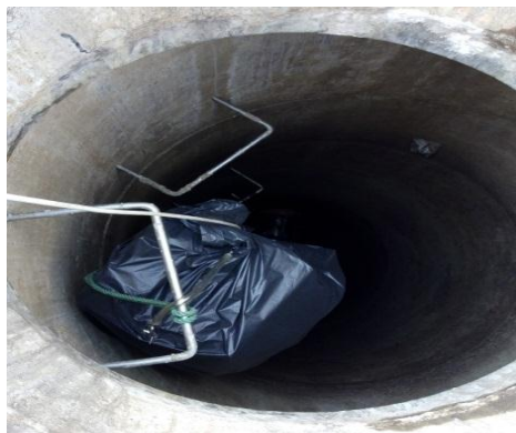
Figure 3.3: Flowmeter hanging at the manhole ladder
