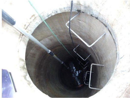
Figure 3.12: The sensor is located at the bottom level of the manhole
