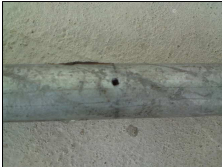
Figure 3.2: Hole as the source of the leak
