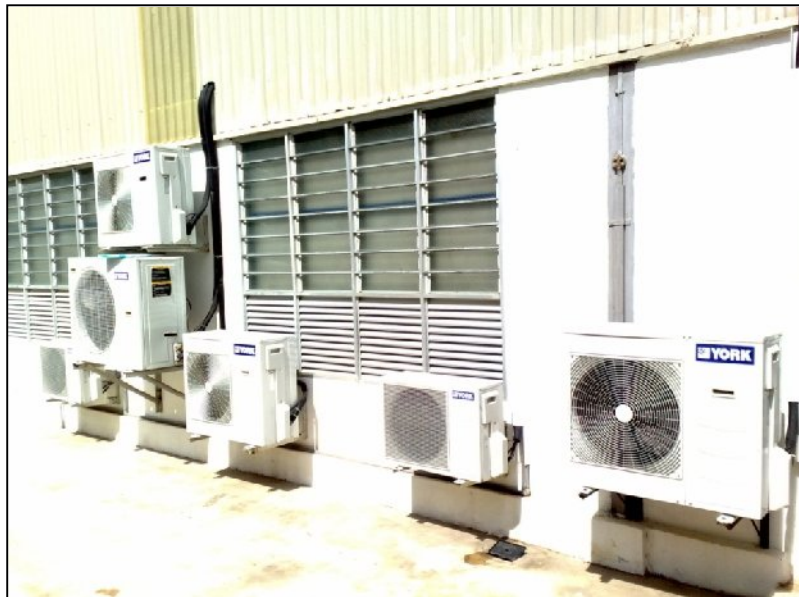
Figure 4.1: A condensing unit of split air conditioning system
