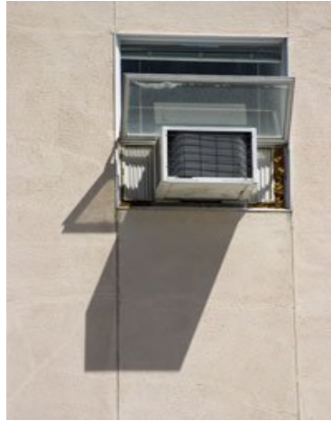
Figure 2.3: Condensing unit (Danny Parker and John Sherwin 2004)
