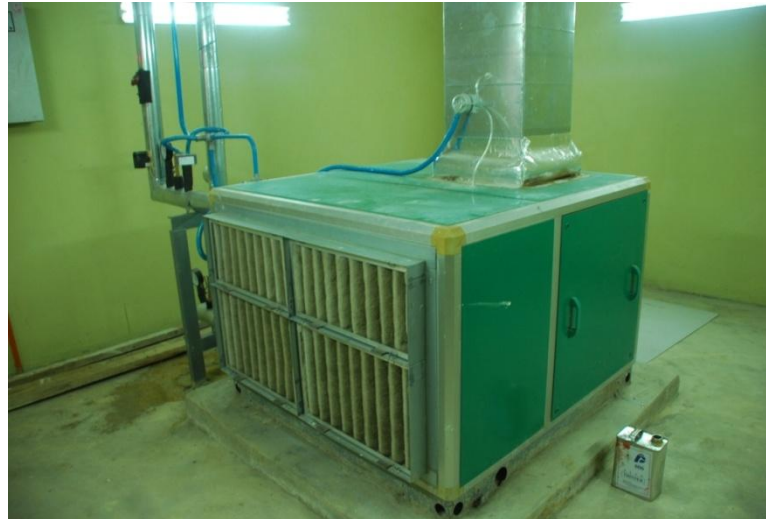
Figure 2.15: Air Handling Unit (AHU) in FKM building
