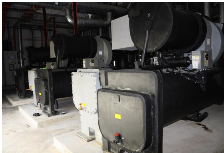
Figure 2.14: Centrifugal chiller in FKM building
