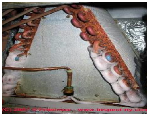
Figure 2.5: Freezing evaporator cooling coil
