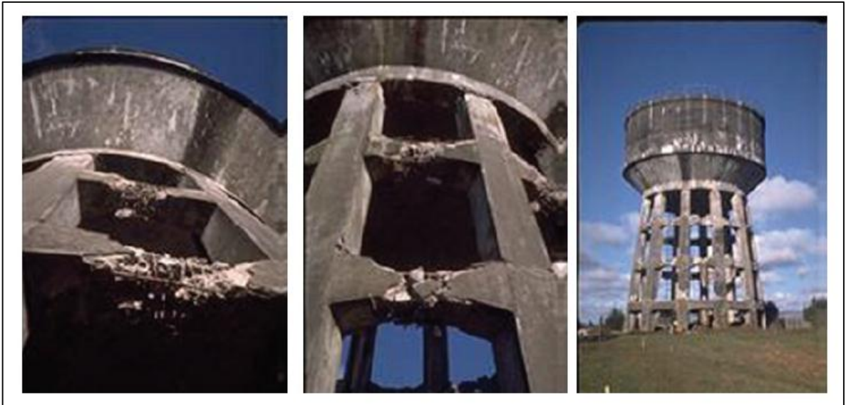
Figure 2.14 : Elevated water tank in Chile earthquake, 1960
