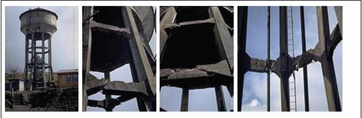
Figure 2.12 : Elevated water tank, 1960, Chile Earthquake
