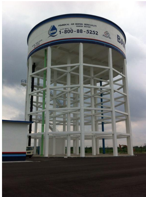
Figure 2.8 : Cylindrical water tank on braced column in Bandar Bestari, Selangor. Sources: perinagasetia.com [Online image]. (2016). Retrieved December 04, 2016 from http://perinagasetia.com/galleries/1177626-project-bandar-bestari-water-tank
