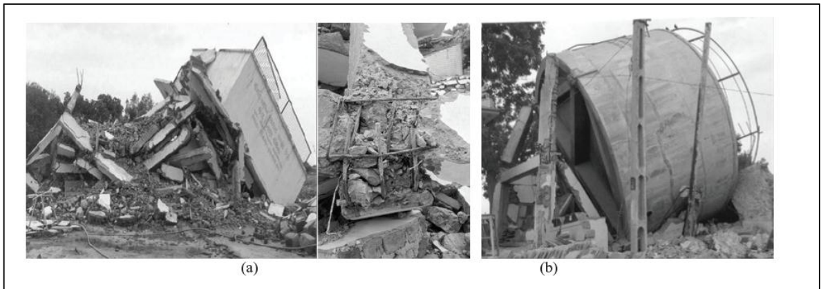
Figure 2.13 (a) - Collapsed slender and weak framed staging of water tanks in Manfera Village; Figure 2.13(b) - Severe damage occurred to elevated water tanks in Bhachau
