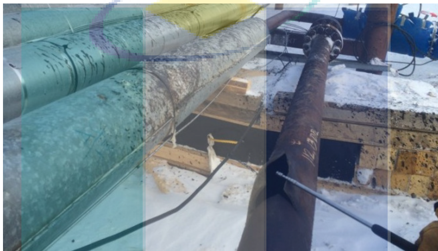
Figure 1.2: Example of a pipeline rupture.
