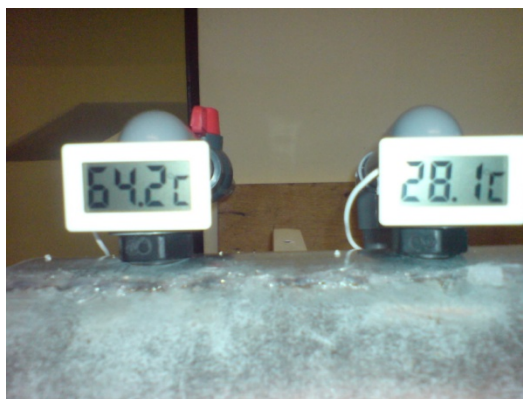
Figure 4.14: Digital thermometer applied to each inlet and outlet.
