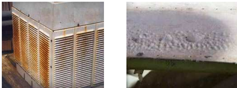
Figure 2.8: Corrosion happened under protective coating. [1]
