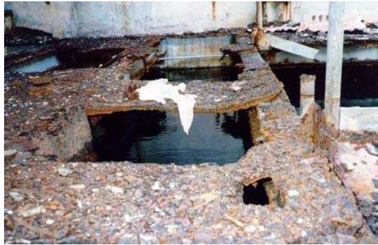
Figure 2.1: Picture show how this corrosion can progress if control measures are not taken. [1]
