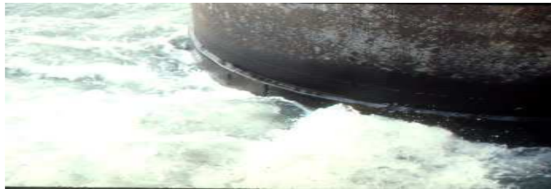
Figure 2.9: The picture shows extra steel added to the bottom of an offshore oil production platform. The one inch of extra steel was added as a corrosion allowance. [1]
