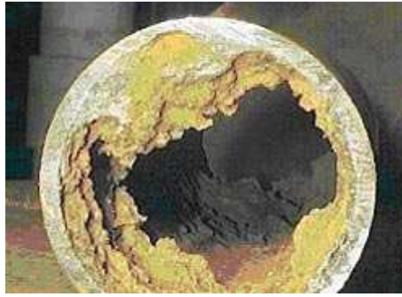
Figure 2.3: Showing the pitting corrosion. [1]
