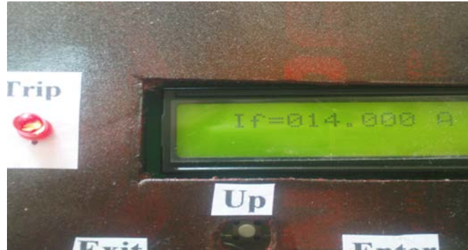
Figure 4.14: LCD shows the fault current
