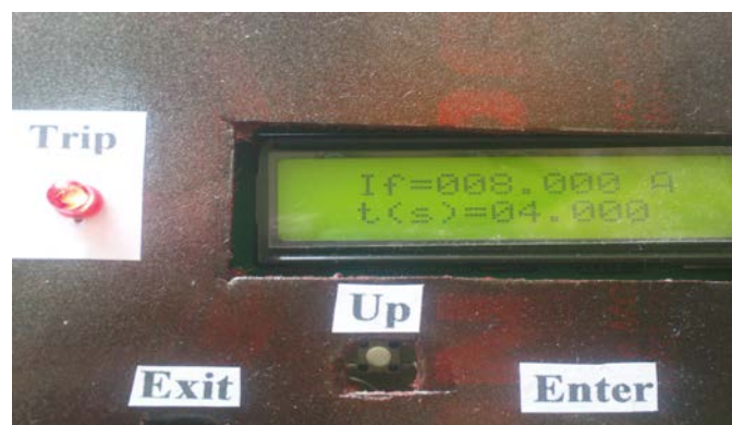
Figure 4.12: LCD display the load current exceeds the I_{>} setting
