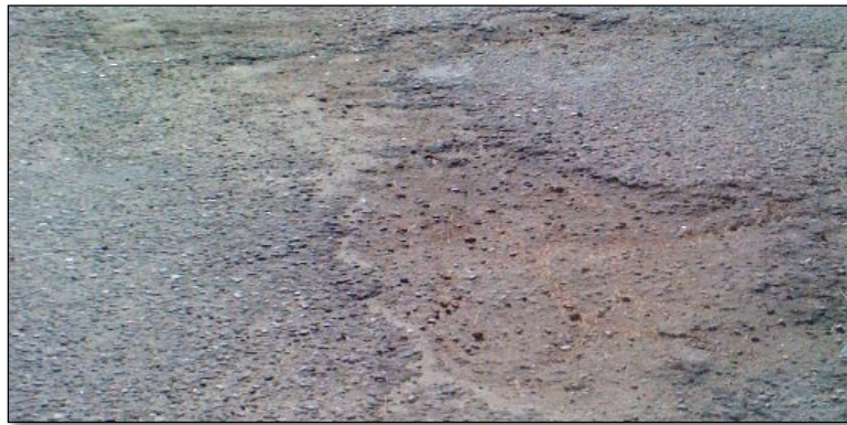
Figure 2.4 Raveling Types Of Road Failure
