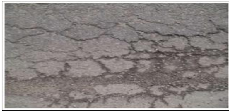
Figure 2.1 Types of road damage (cracking)
