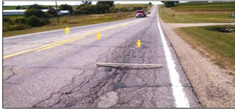
Figure 2.2 Grade depression damage
