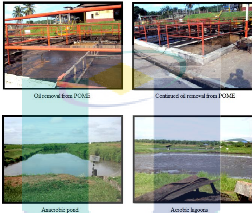
Figure 2.3: Working POME ponding system in oil palm mill
