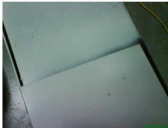
Figure 4.6: Incorrect position of door
