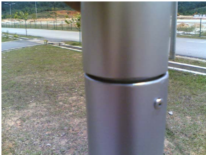
Figure 4.7: Gap between two materials after assembly.
