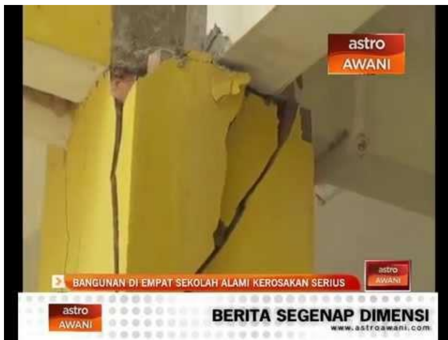
Figure 6.2: The implications of undone scheduled maintenance works
