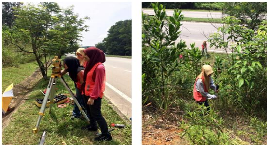
Figure 3.2 Surveying works is done to measure the height and length of the slope
