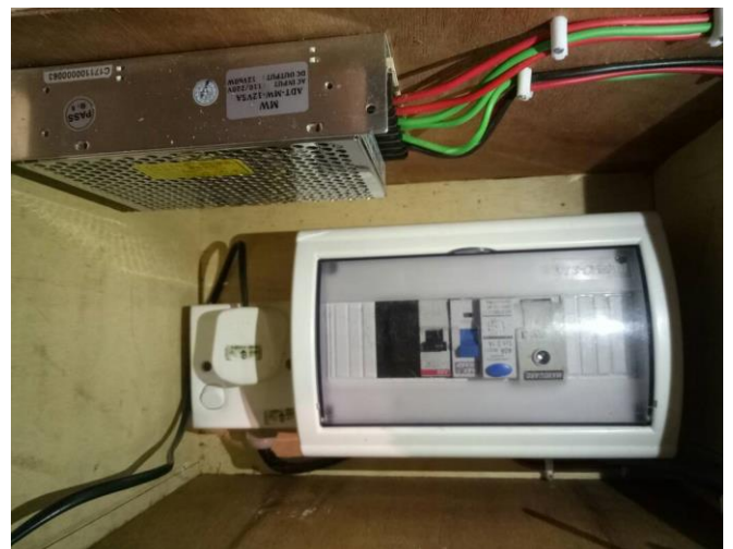
Figure C4: Distribution Fuse Box
