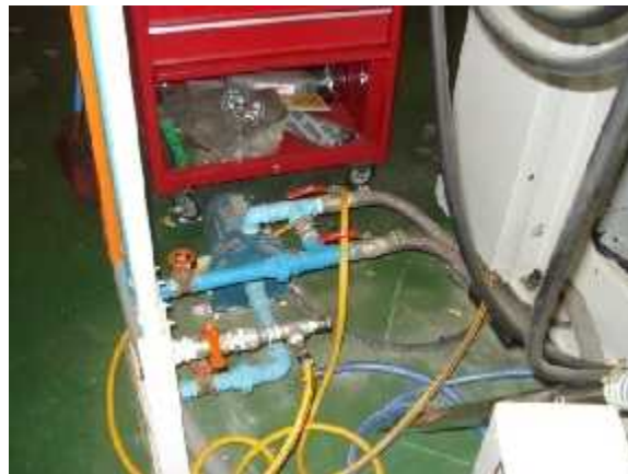
E. Water pipe that flow to Mould to cool is down.
