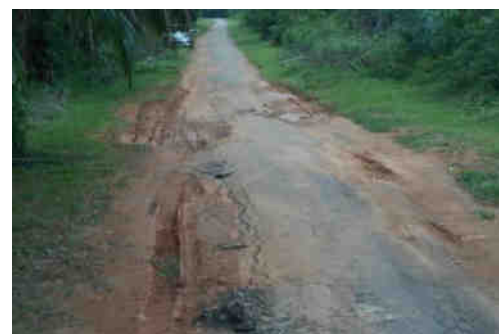
Fig. 2: Potholes and cracking
