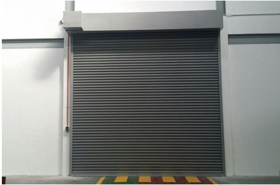
Figure 5.6: Fire resistant roller shutter
