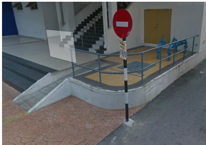
Figure 4.9.4. b: Handrail is not provided at the ramp but the kerb is providing
