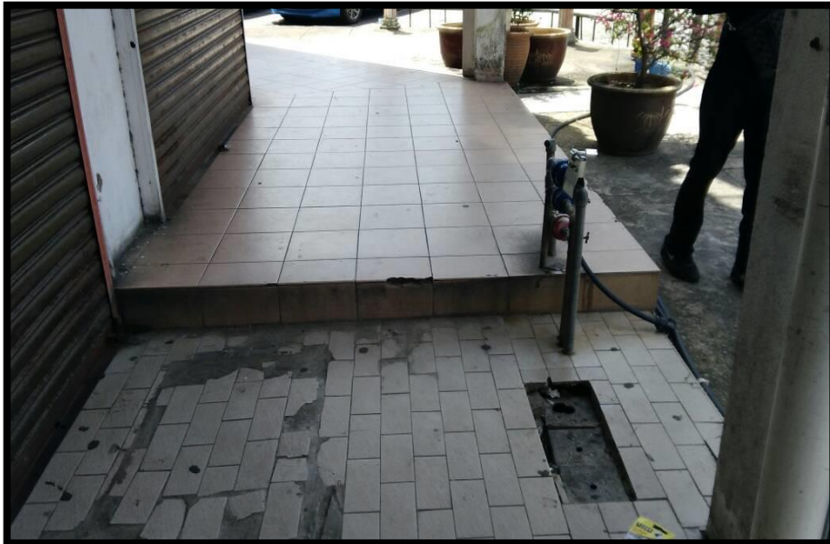
Figure 4.8.4.a: Improper kerb ramp
