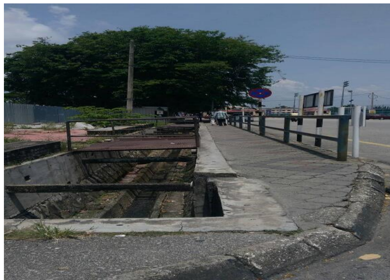
Figure 4.9.1a: Handrail only provided at one side and no passing space and improper drain cover
