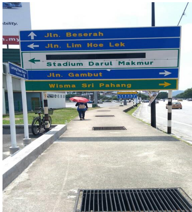
Figure 4.9.3.a: No handrail provided, no passing space and drain cover is wrong direction
