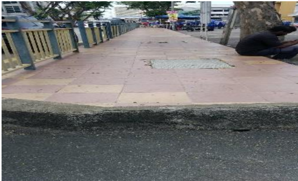
Figure 4.9.2.a: Handrail only provided at the side of the walkway
