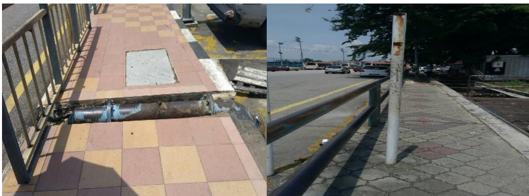
Figure 4.6.1.d: Barrier at the middle of walkway
