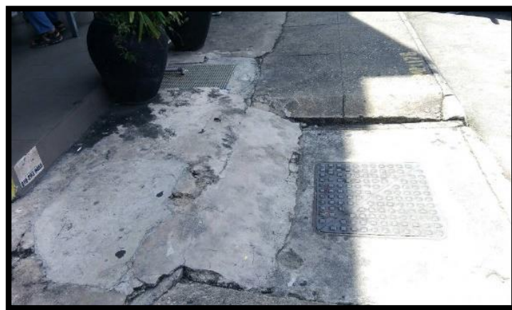
Figure 4.9.4.c: Not proper maintenance of the drain cover
