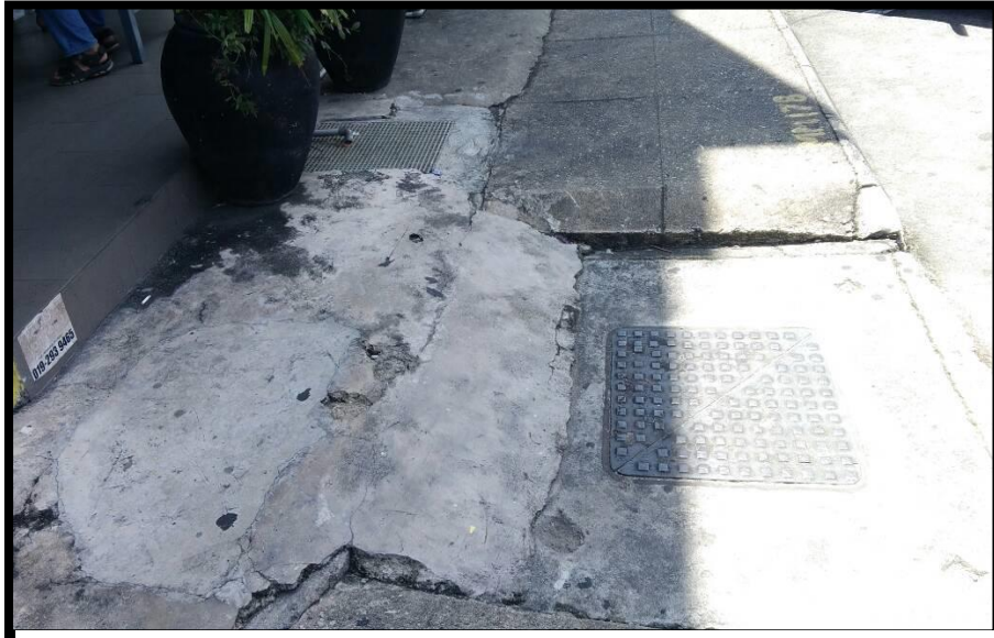
Figure 4.8.4.b : No kerb ramp provided
