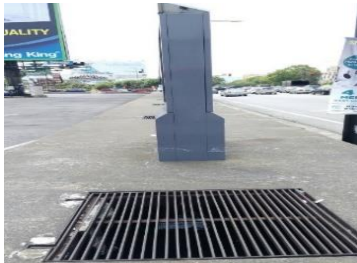
Figure 4.6.3.c: Litter bin that blocking the path of the walkway
