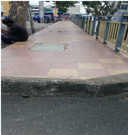
Figure 4.8.2. a: No kerb ramp provided
