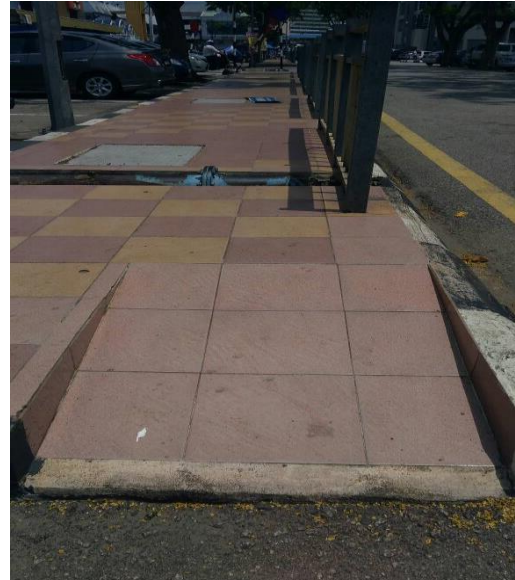
Figure 4.8.1.b : Improper kerb ramp
