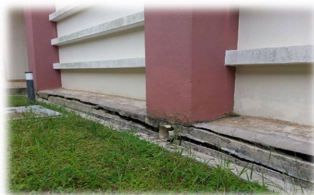
Figure 3.10 Cracked Around the Building Structure
