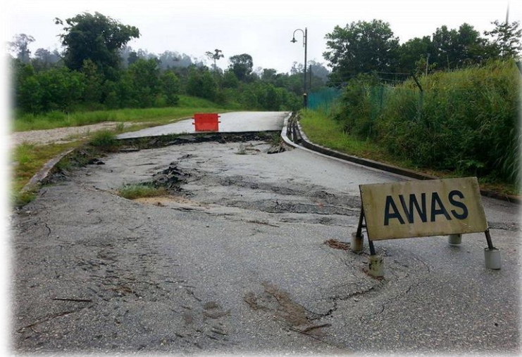
Figure 3.11 Collapsed of Road along the Slope
