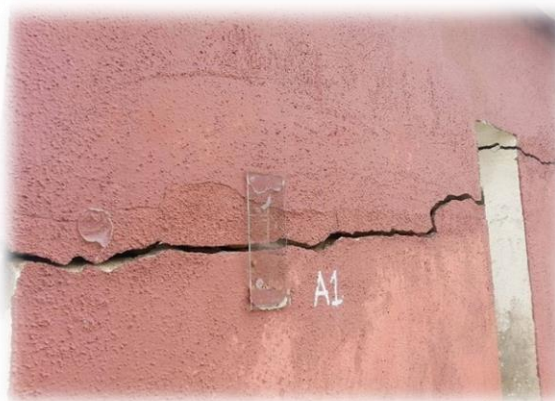
Figure 3.6 Cracked on the Wall of Building
