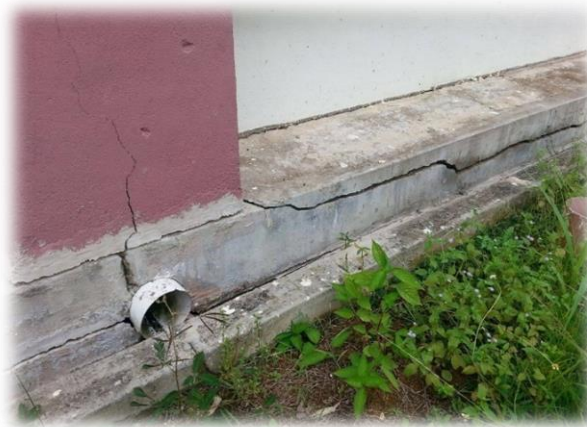
Figure 3.5 Cracked Around the Building Structure
