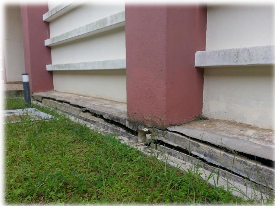
Figure 1.2: Cracked formed on the building structural
