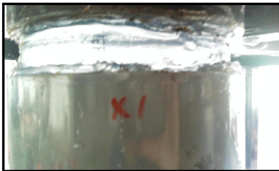
Figure B.2: The mark place of leaks
