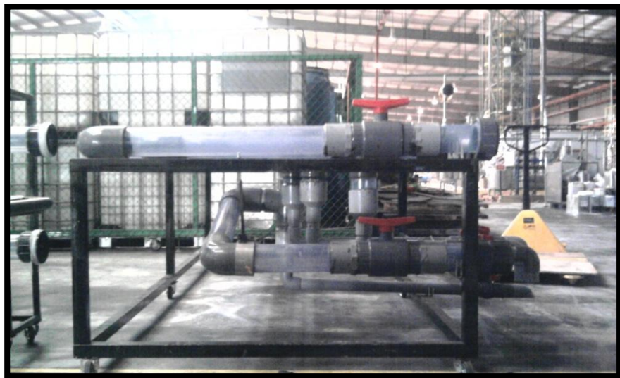
Figure A.12: Front view of solar receiver
