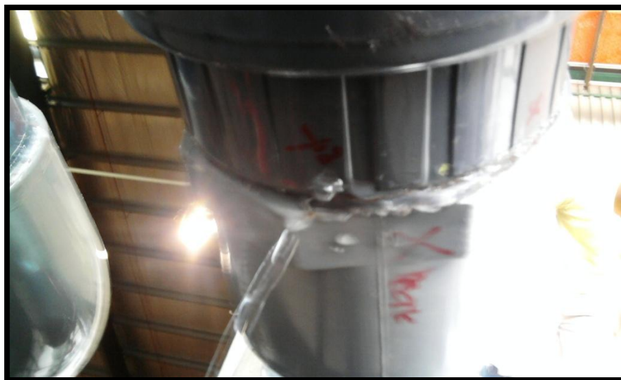
Figure B.1: The leaks at the photobioreactor
