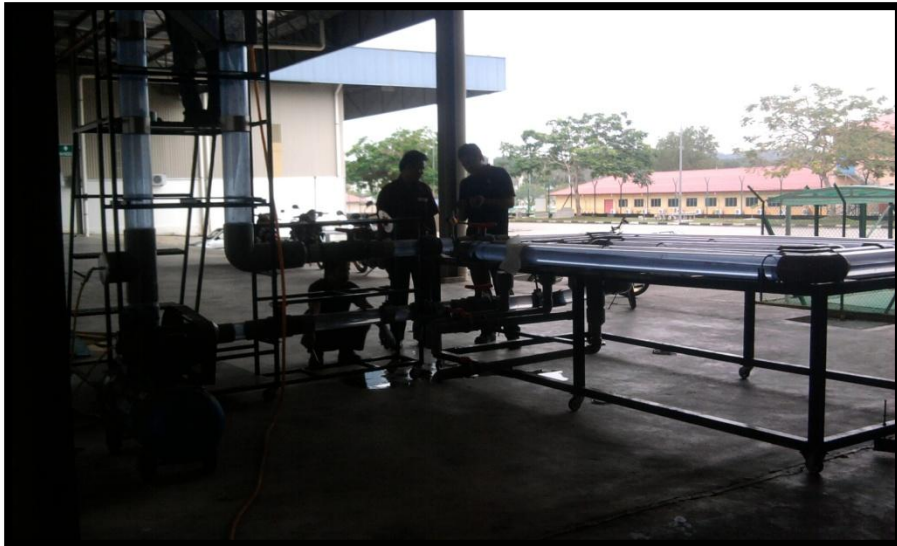
Figure A.19: Checked the leaking
