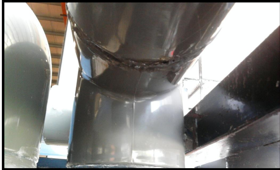
Figure B.3: The part of leak with glu
