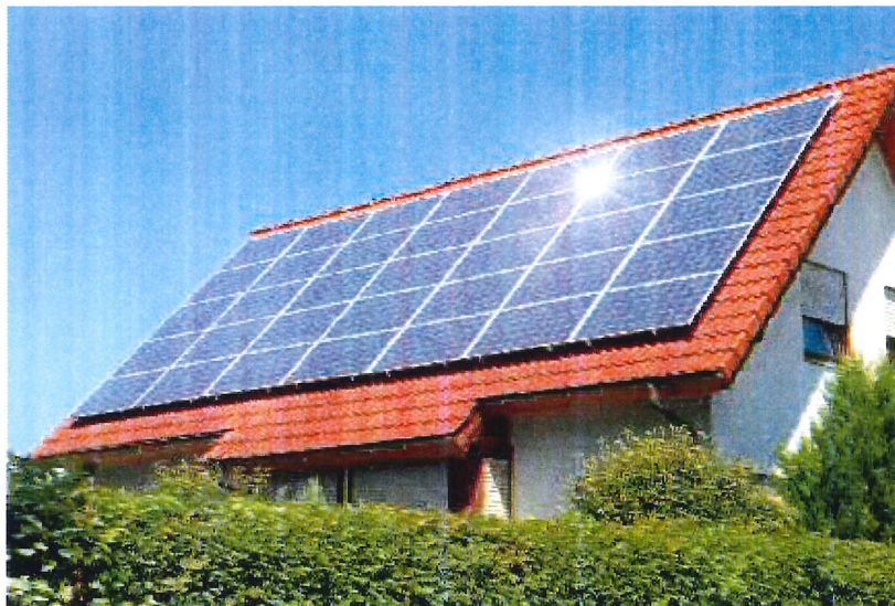
Figure 2.1: Fix-mounted solar panel fixed on roof
