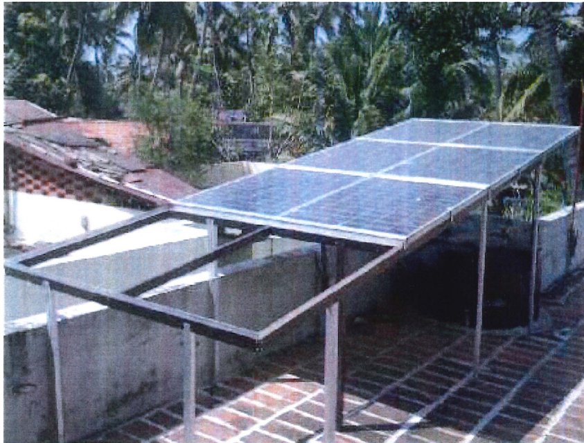
Figure 2.4: Solar panel being fix-mounted on ground by solar mounting structure
