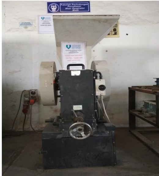
Figure 3.5: Crushing machine that used to pulverize palm oil clinker
