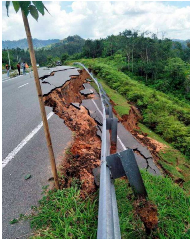
Figure 1.1 Landslide at the Cameron Highlands-Sungai Koyan road Source: m.thestar.com.my/
