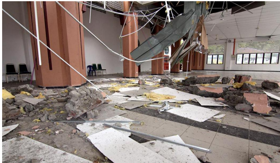
Figure 2.3 A section of the ceiling of Ranau District Mosque that collapsed due to the earthquake ( http://www.theborneopost.com/2015/06/07/psychosocial-team-in-ranau-to-help-victims/ )
