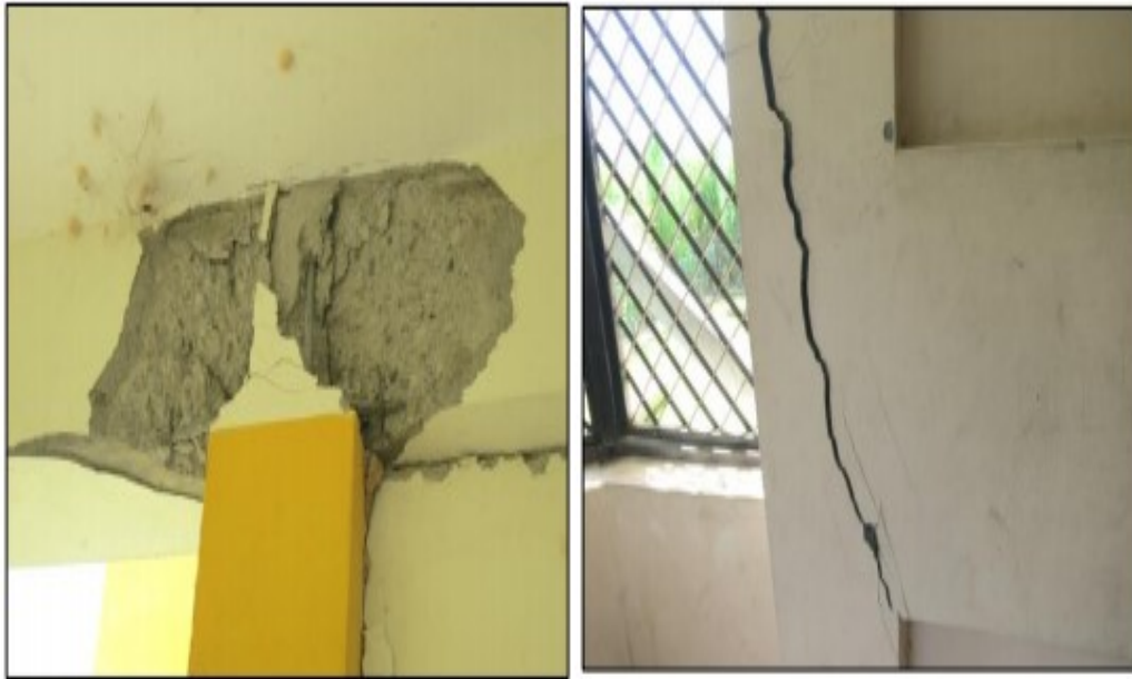
Figure 2.2 Damage on RC beam-column joint due to 2015 Ranau earthquake (Majid et. al., 2017)
