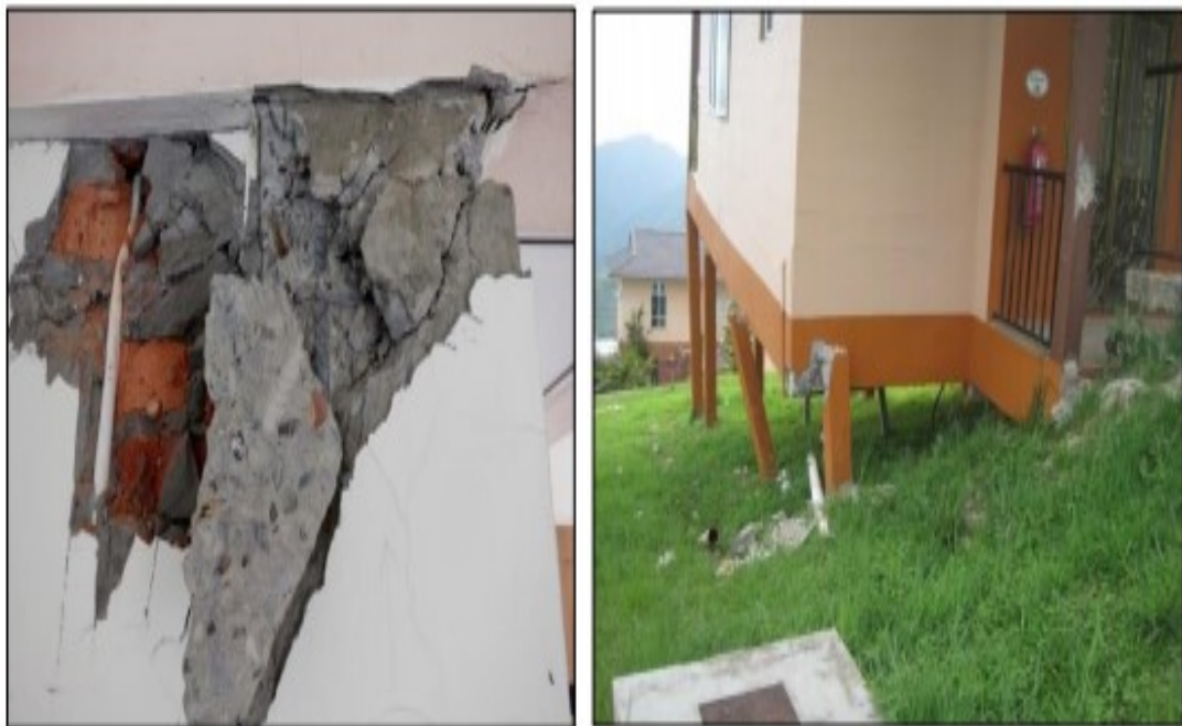
Figure 2.1 Significant damage on RC column due to 2015 Ranau earthquake (Majid et. al., 2017)
