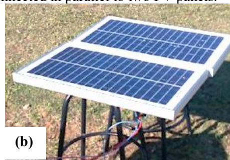
PV panels position (parallel to the ground)
