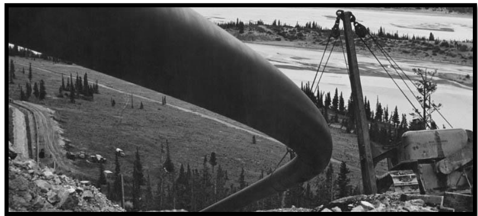
Figure 2.1: Transmission pipeline transport crude oil from Edmonton, Wiscinsin, USA (Hays, 2015)
