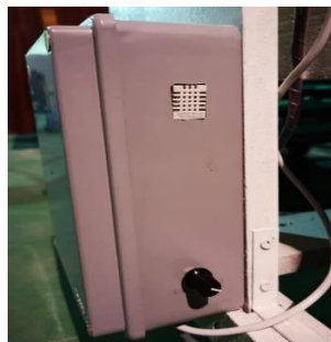
Figure 4.15 Side view of the electrical box
