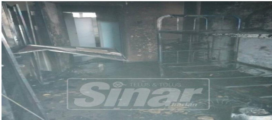
Figure 1.2: Fire Accidents in Kolej Kemahiran Johor (Sinar Harian Online 2018)
