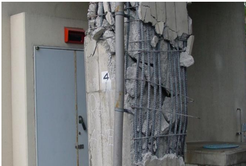
Figure 2-3: The Example of Defective Workmanship
