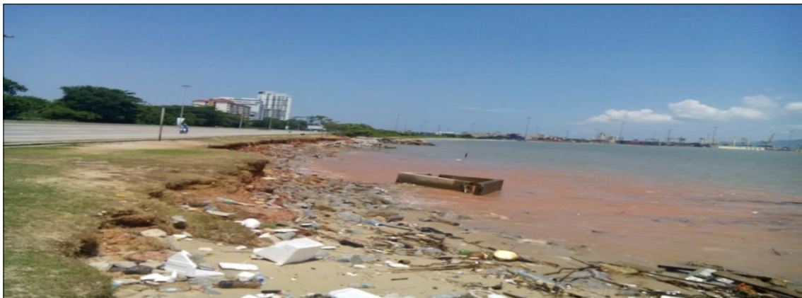
Figure 1.2 Coastal erosion at Butterworth Outer Ring Road, Penang
