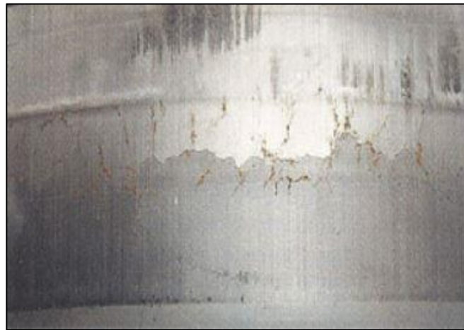
Figure 2.8 Austenitic stainless steel subject to stress corrosion cracking
