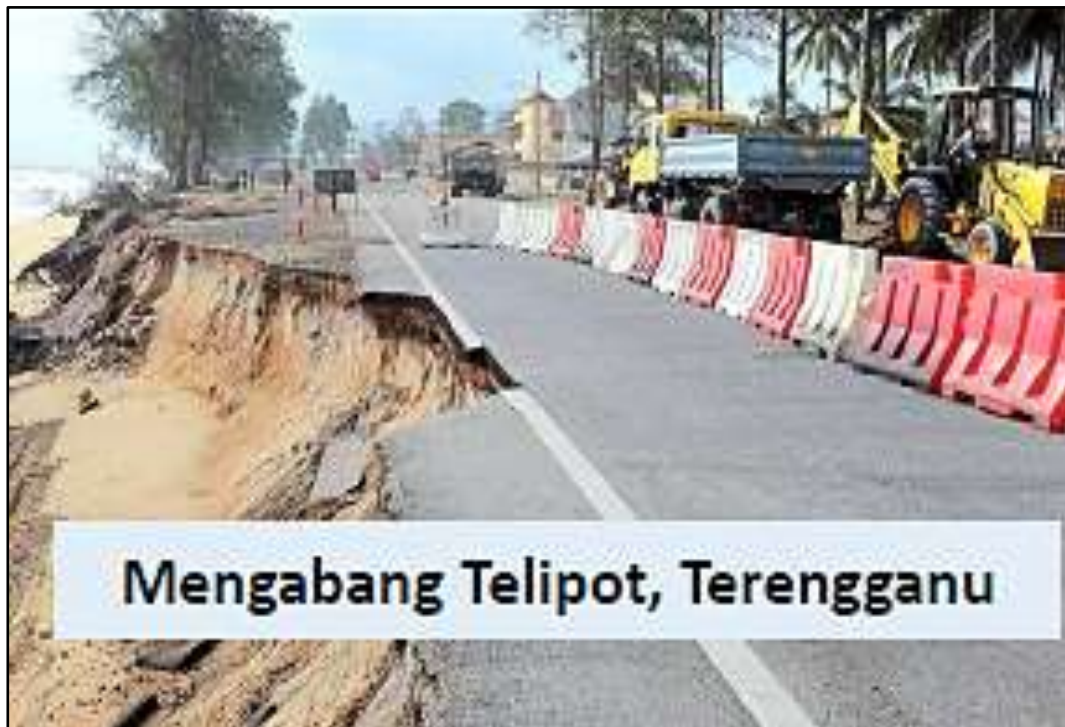
Figure 2.10 Damage and Erosion of Main Road due to Sea Level Rise at Mengabang Telipot, Terengganu
